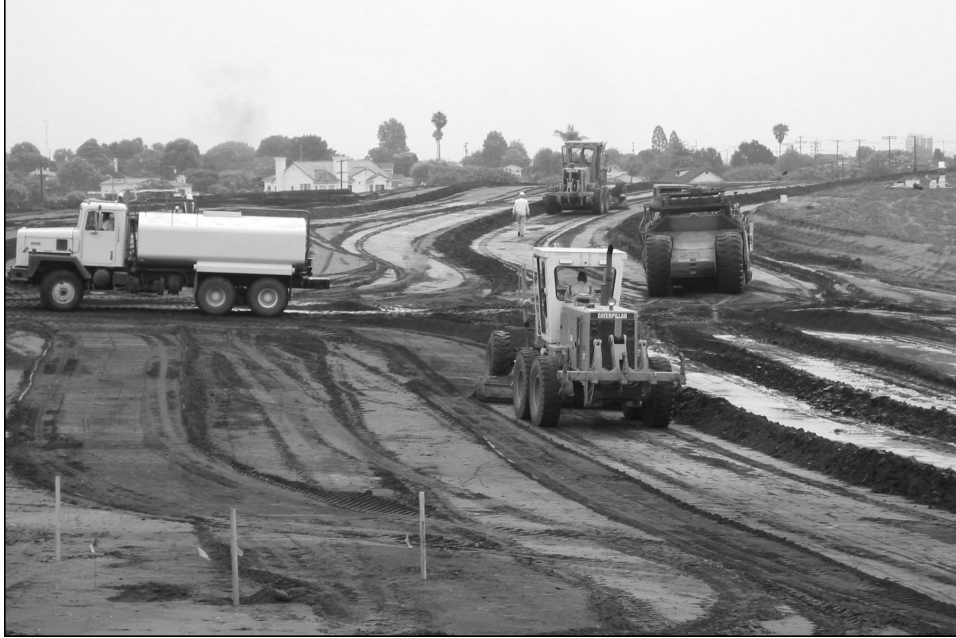
Figure 4.6. Grading and monitoring operations at West Bluffs in the summer of 2003. Heavy equipment includes two graders, a bottom-loading scraper used to load the earthen windrows, and a water truck used for dust control. Archaeologists monitored the grading operation for exposed cultural deposits, artifacts, and features.
