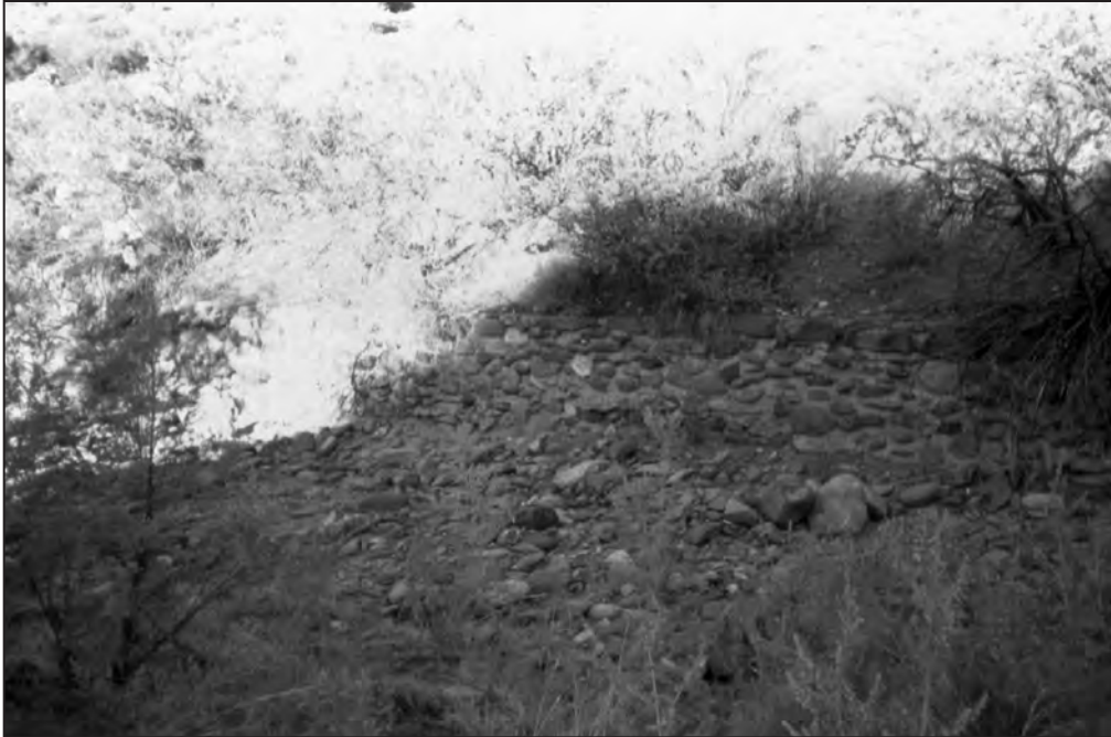
Figure 173. Masonry retaining wall along the old FH 9 roadbed near the Gold Creek Bridge.
