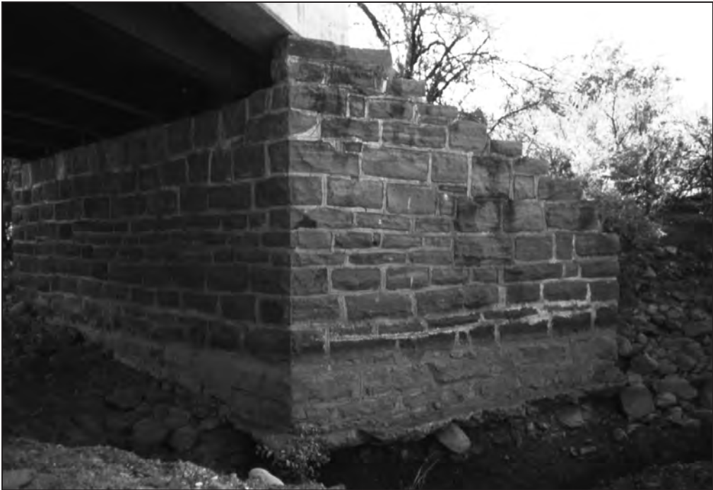
Figure 172. Detail photograph of stone and concrete abutments of the old Gold Creek Bridge.
