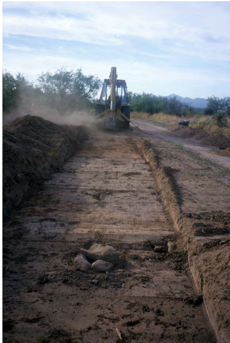
Figure 78. Photograph of backhoe excavating narrow and shallow stripping units in Locus D during Phase 1.
