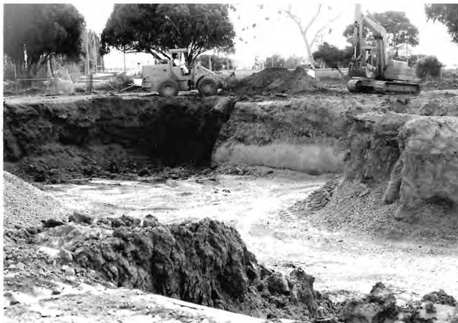
Figure 44. Photograph of John Deere backhoe and front-end loader working in tandem during soil remediation on Bay City Metals lot.
