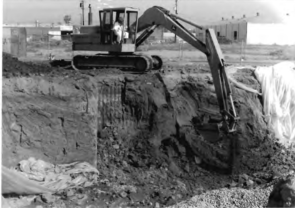
Figure 43. Photograph of John Deere backhoe removing soil from Avis lot for remediation (note the Marina Storage building in upper right corner).
