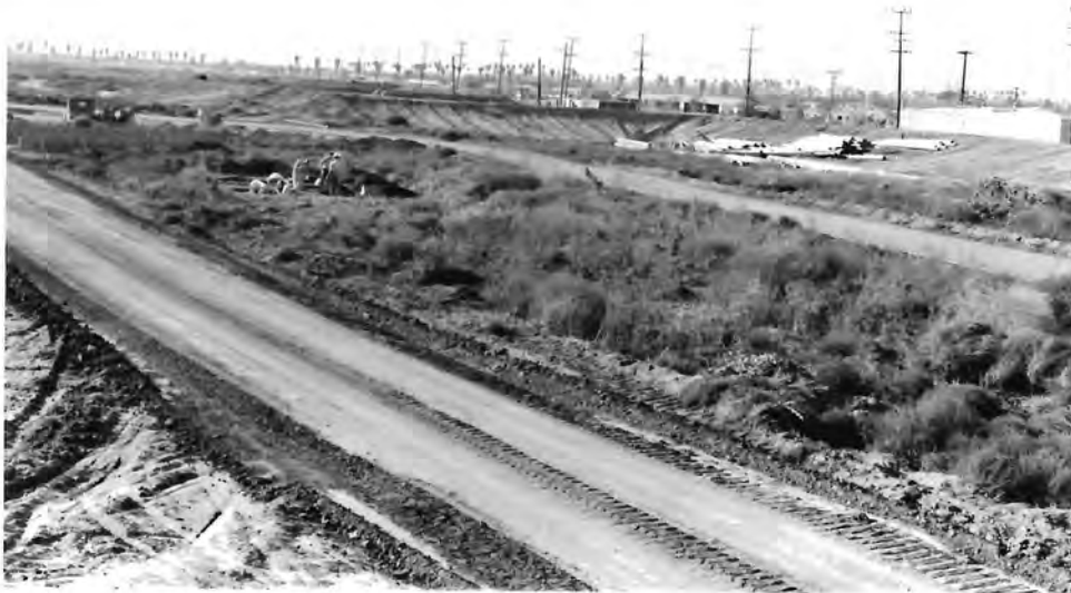
Figure 32. Second UCLA excavation unit, looking north. Note: Transmission line marks the railroad right-of-way and the white building on the right side of photograph is the Bay City Metals Building (Photograph courtesy of Keith Johnson).
