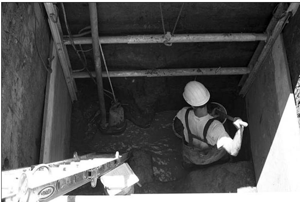
Figure 148. Photograph of excavation within a deep unit at LAN-62 Locus A. Note the hydraulic shoring of the EU and the water pump in the corner of the unit to extract water seepage because the unit was excavated below the water table.
