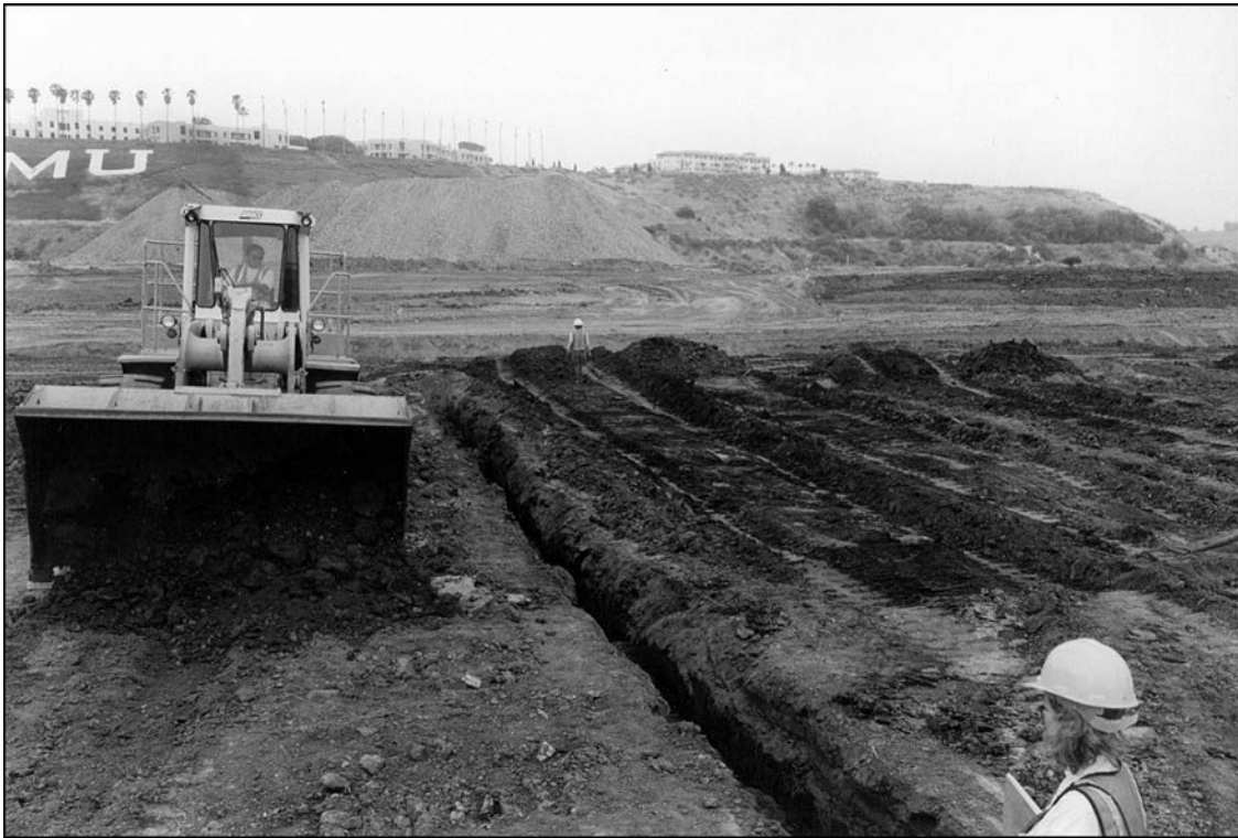
Figure 253. Photograph of the removal of overburden and trench excavation during the second testing phase at LAN-1932, view to the south.
