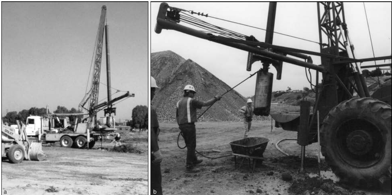
Figure 13. Bucket augering: (a) overview of the auger mounted on the rig and (b) close-up of auger sample collection.
