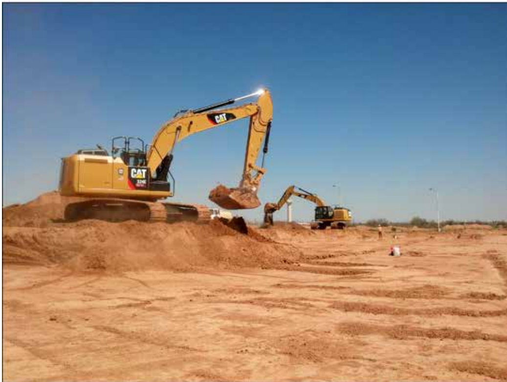
Figure 10. Heavy equipment utilized during mechanical stripping: (top) an excavator, a front-end loader, and a water truck, view to the west, and (bottom) two excavators stripping two adjacent MSUs.
