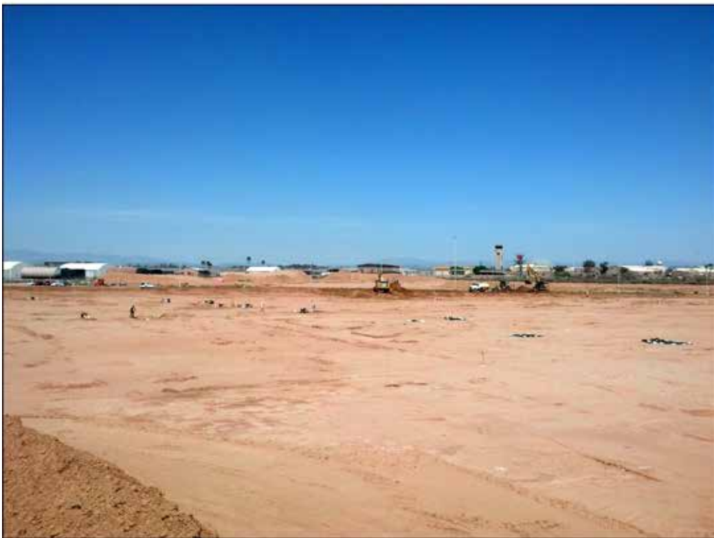
Figure 12. Photographs of Phase 2 excavations: (top) Area A, view to the southeast, and (bottom) Area B, view to the northeast.
