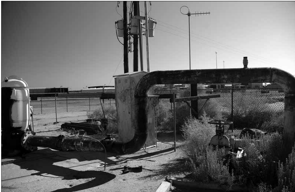
Figure 259. Pump and water-distribution line, view to northeast, August 4, 2010.
